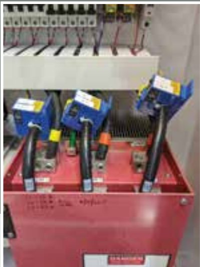
Ammeters and current transducers
