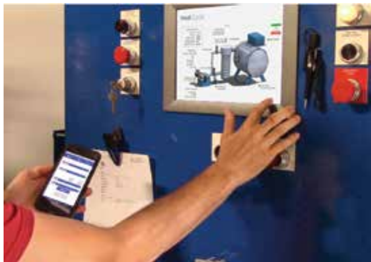
Fig. 2. Integrated controls with SCADA provide quick access to information and unique data-capture capabilities.
