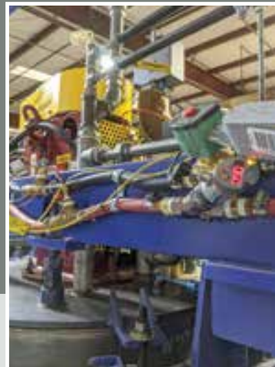
Flow and pressure monitoring
